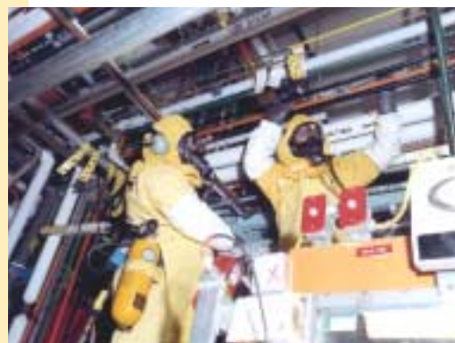
Workers drained and removed more than 11 miles of piping containing plutonium solutions.
