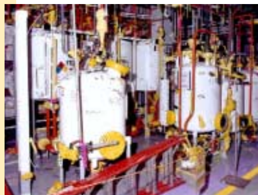
In 1995, tanks containing plutonium solutions.
