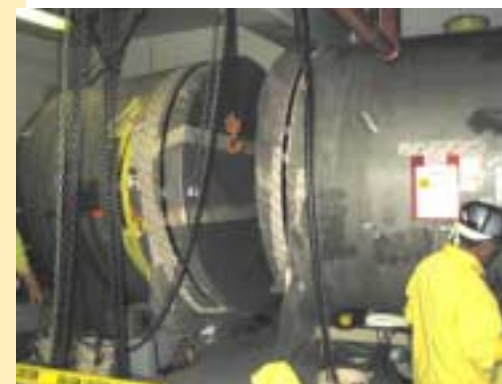
Large tanks also had to be cut into pieces to fit in radioactive waste shipping containers.
