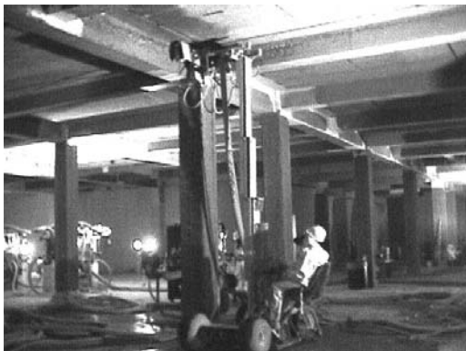
Figure 3. TMR Locally Operated Ceiling Unit
