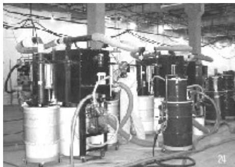
Figure 5. WSS Systems at RFETS
